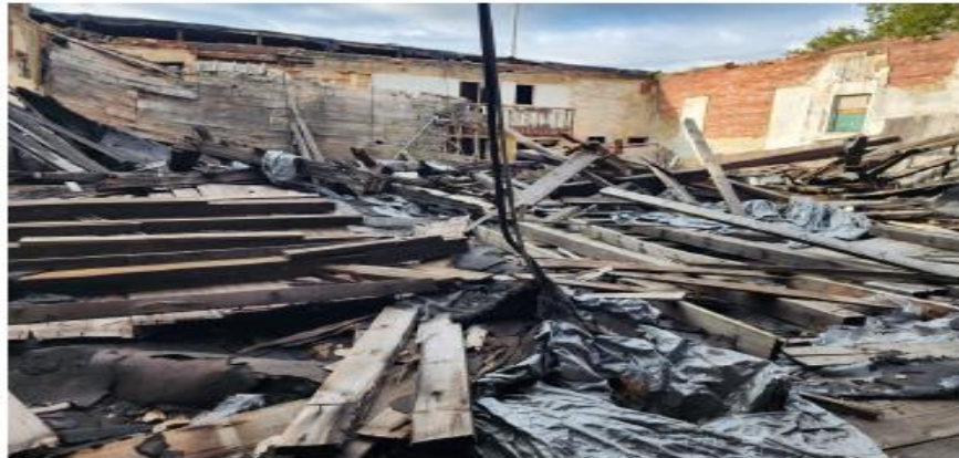
View of the interior of the theater & dance hall with collapsed roof.
