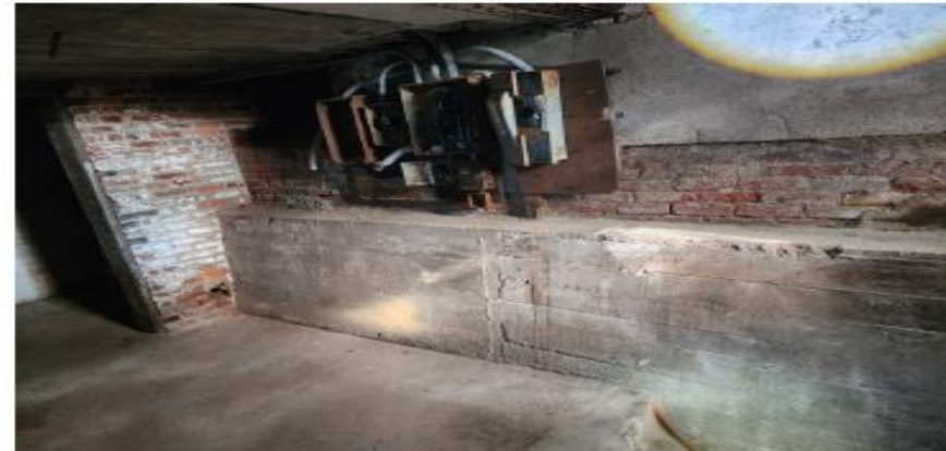
View of the electrical utility area in the basement.
