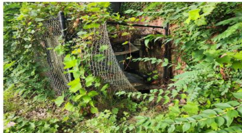
View of a vandalized HVAC unit on the east side of the structure.
