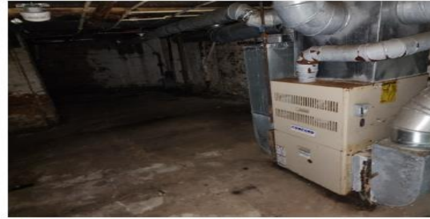
View of a natural gas fired furnace in the basement.
