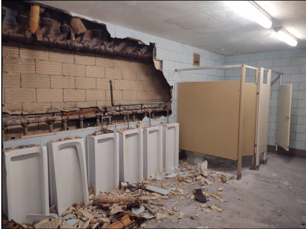
5 : 5 Substantial damage to restroom to remove copper piping.
