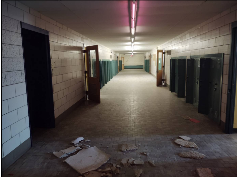
29 : 29 Representative view of third floor hallway. Damage from vandalism is apparent.
