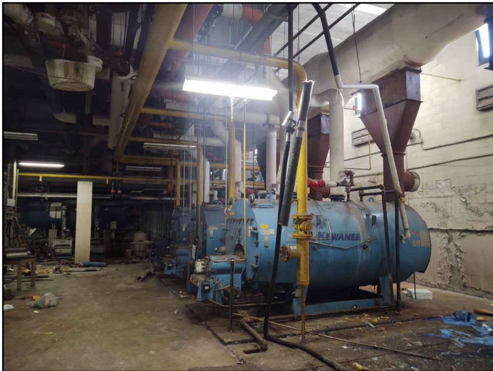
10 : 10 View of boiler room. Three boilers.
