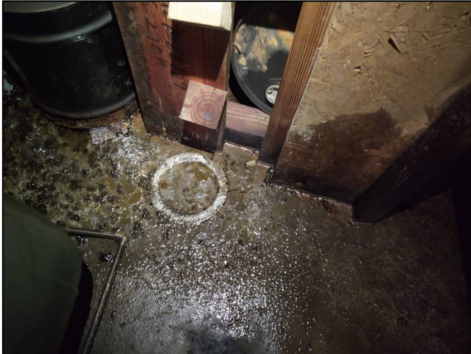
17 : 17 Accumulation of oil on floor behind chiller unit.
