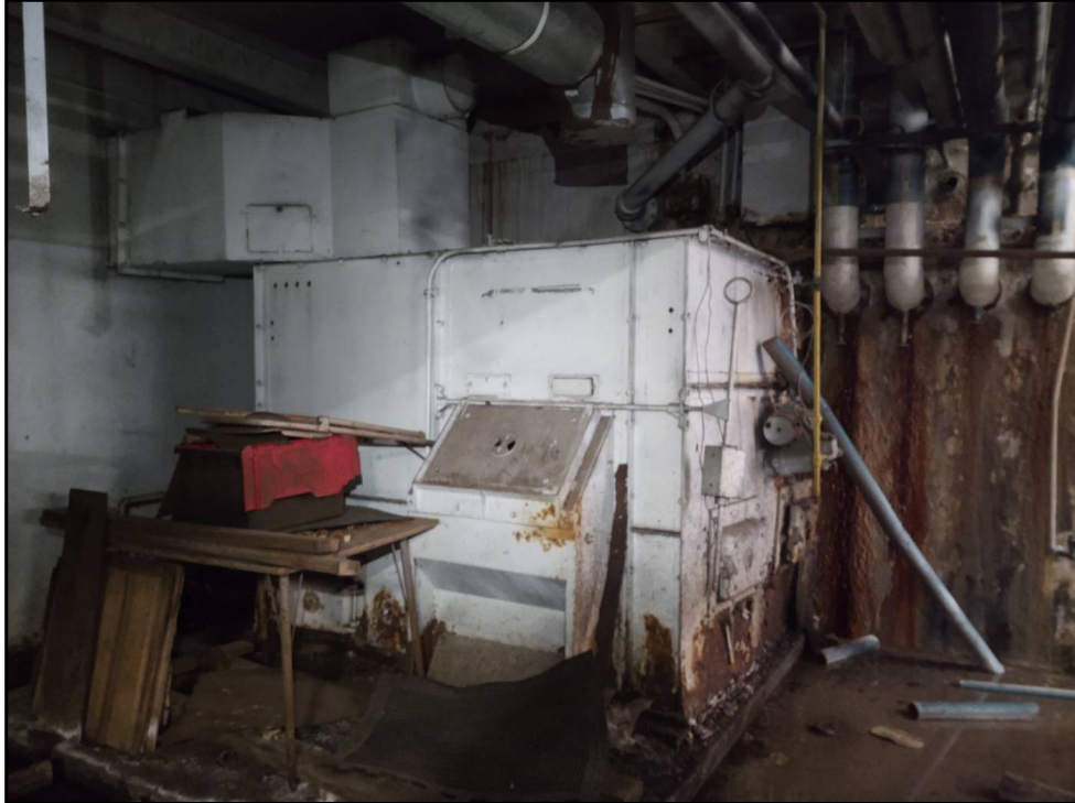
19 : 19 Incinerator present in boiler room. Most recent use is unknown.
