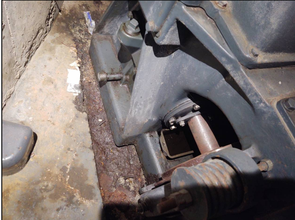
21 : 21 Oil leaks from elevator motor are apparent.
