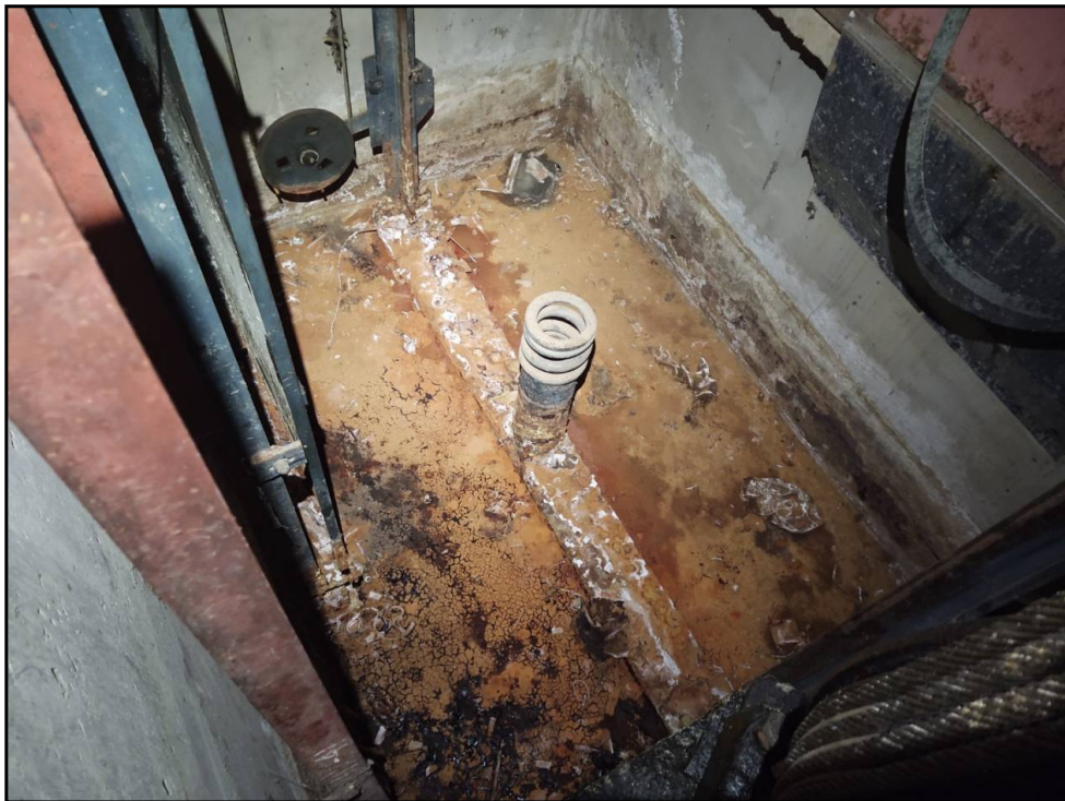
22 : 22 Migration of oil from elevator motor, across the floor, to bottom of elevator shaft is apparent.
