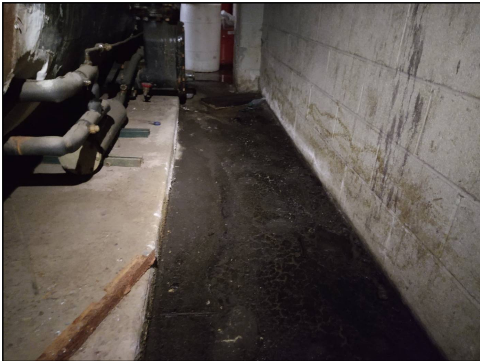
14 : 14 Accumulation of caked oil on floor behind chiller unit.
