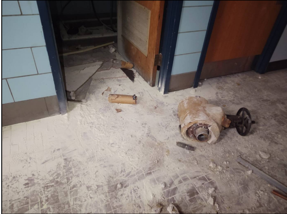
31 : 31 Representative view of damage to mudded pipe fittings by vandals.
