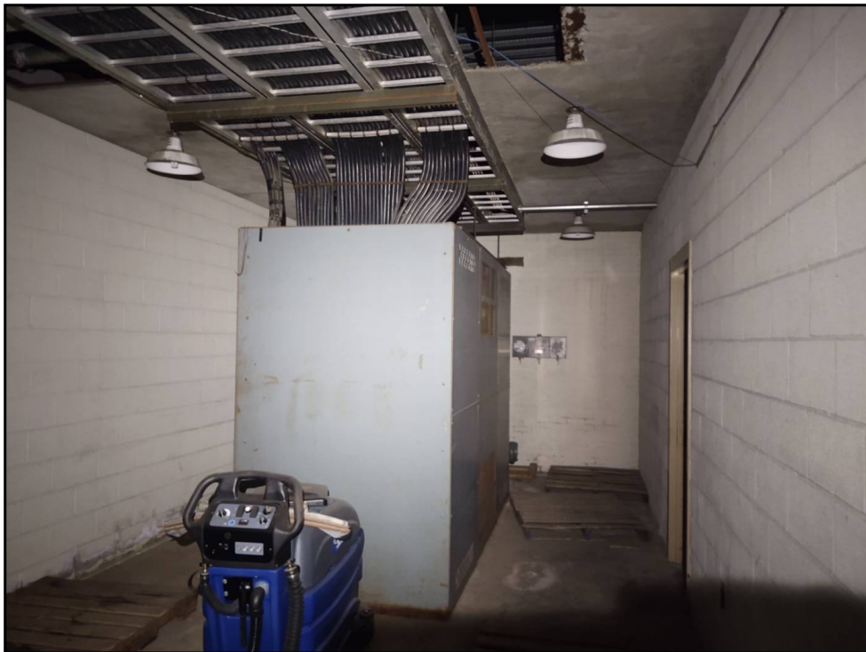
24 : 24 Original transformer / electrical switching equipment is still present.
