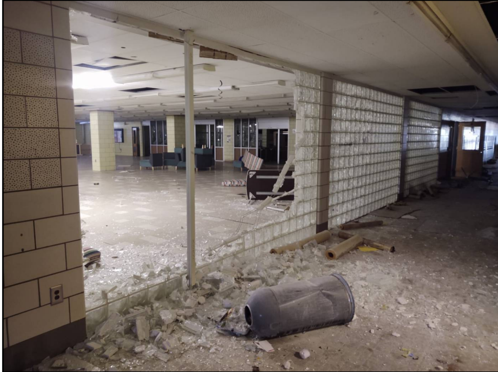
25 : 25 View of vandalism in cafeteria area.
