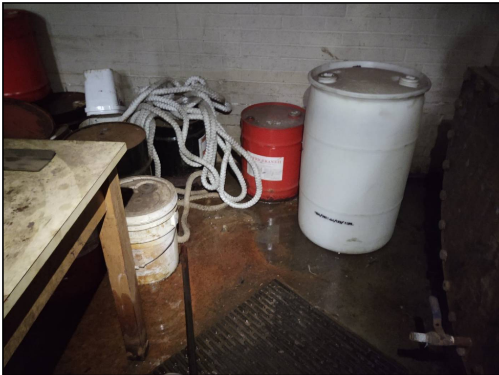
16 : 16 Improperly stored, and unlabeled containers of chemicals on floor behind chiller amongst accumulation of rainwater/ groundwater infiltration on floor.
