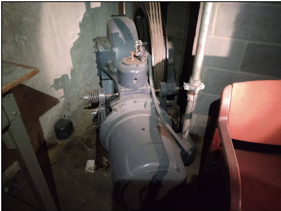
20 : 20 Elevator motor is original to building. Documentation with unit indicates manufacture in 1960.
