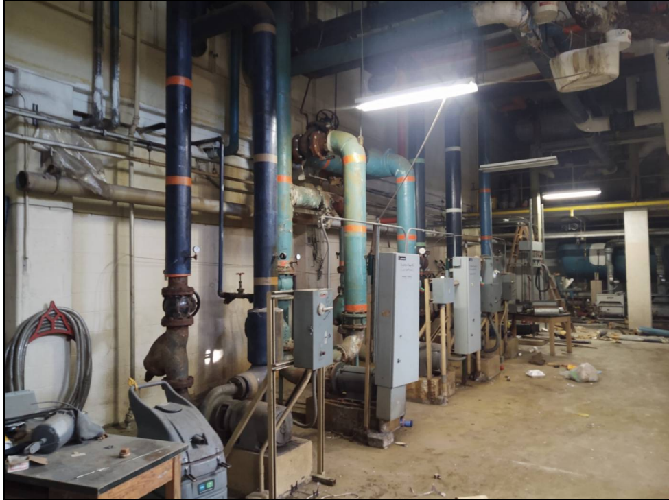
11 : 11 View of high-pressure steam, and low pressure steam return pumps.
