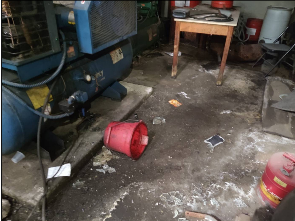
15 : 15 Improperly stored chemicals on floor between chiller unit and air compressor. Staining on concrete floor apparent.
