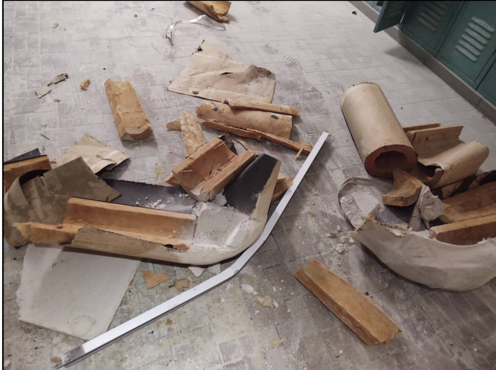
3 : 3 Vandals have removed most of the copper steam and water piping from the building. Mudded pipe fittings and elbows are likely ACM.
