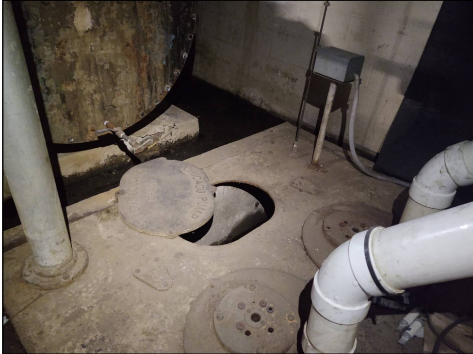
13 : 13 Make up water sump behind chiller
